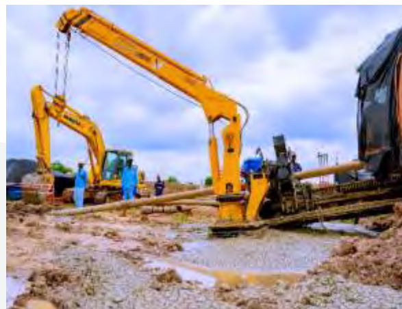
AKK Gas pipeline Sector 2
